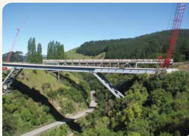
State Highway 2 Matahorua Gorge Realignment between the Hawke's Bay and Gisborne regions.
