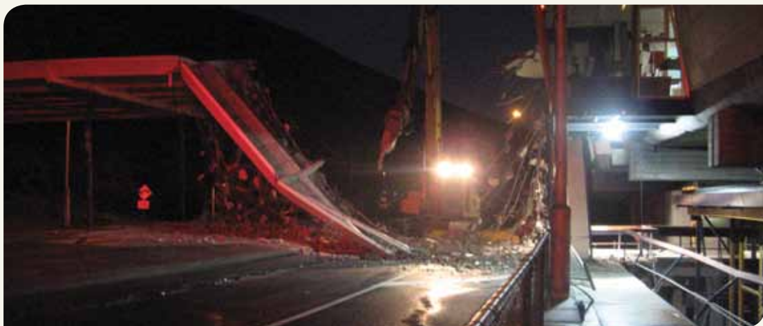
The Lyttelton Tunnel canopy destroyed by the quake.
