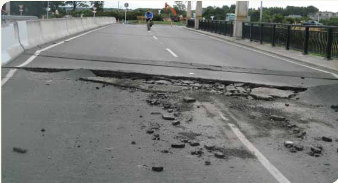
Quake damage to the ANZAC Drive Bridge.
