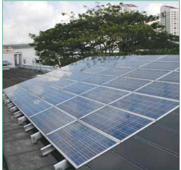
Figure 4: PV array mounted at an angle on the building roof top
