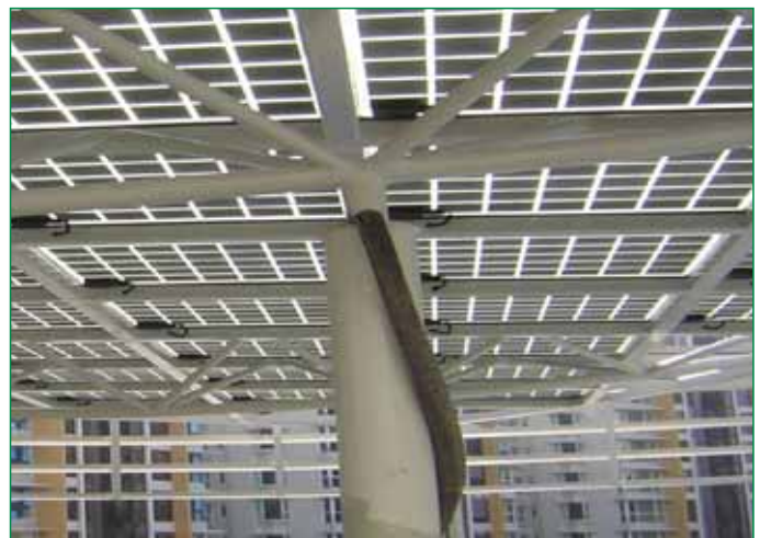
Figure 6: PV modules integrated into skylight canopy (Courtesy of Savannah Condominium)
