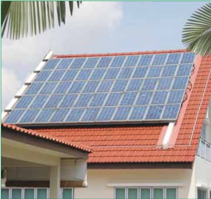
Figure 3: Roof Mounted PV System (Courtesy of Interlink Power System)
