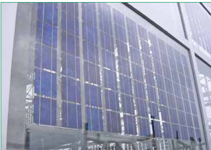
Figure 5: PV modules integrated into facade (BIPV) (Courtesy of Biopolis)
