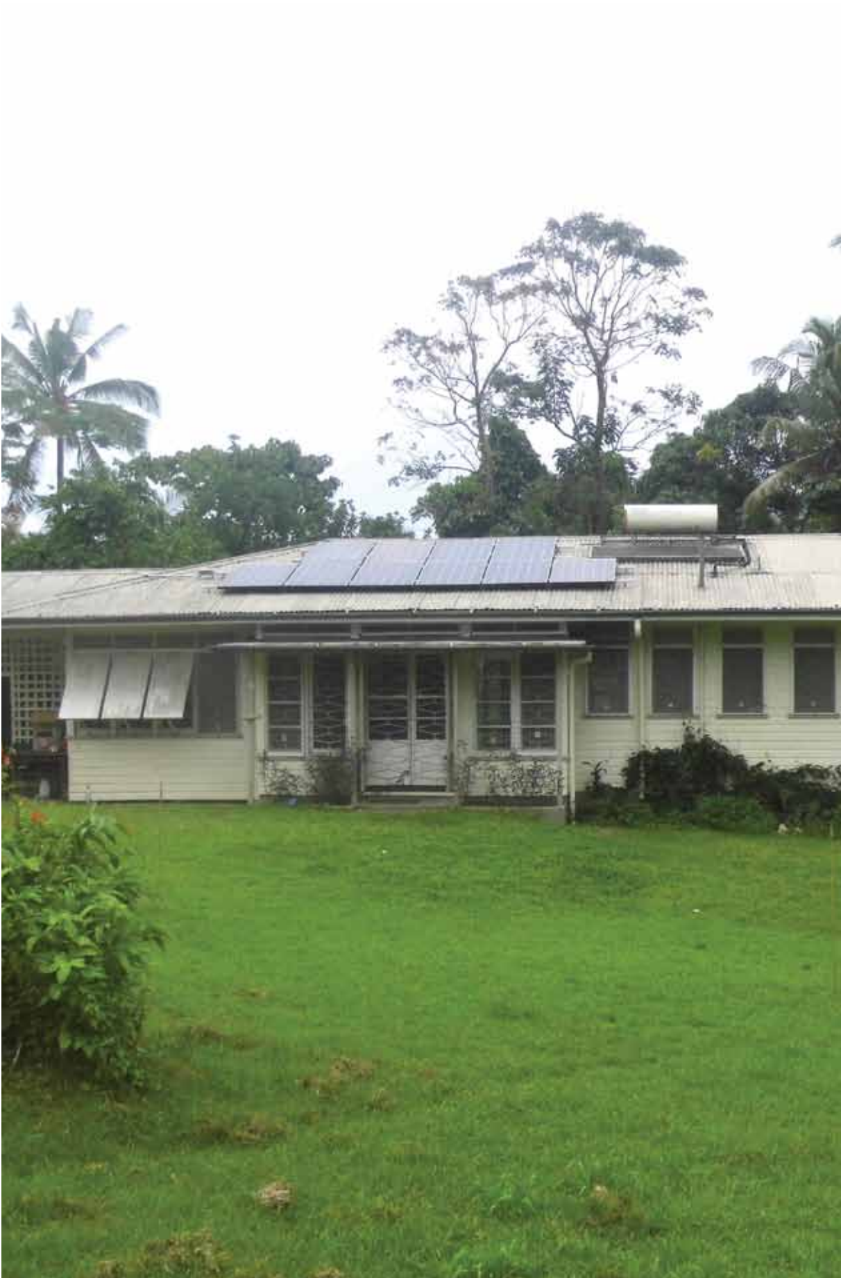
GCPV and solar water heater Photo: Government of Fiji
