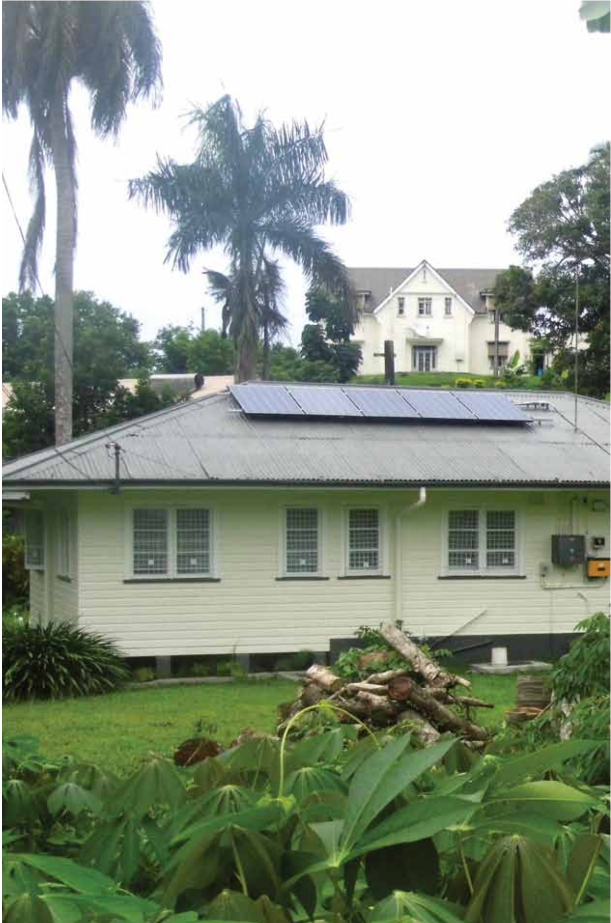
Grid connect PV at Government quarters Photo: Government of Fiji
