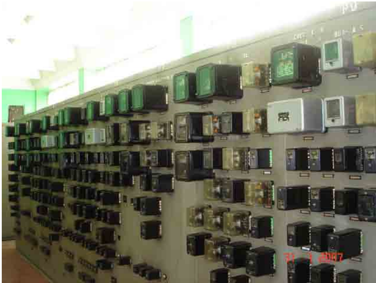
Figure 2: Darunta (Jalalabad) Control System
