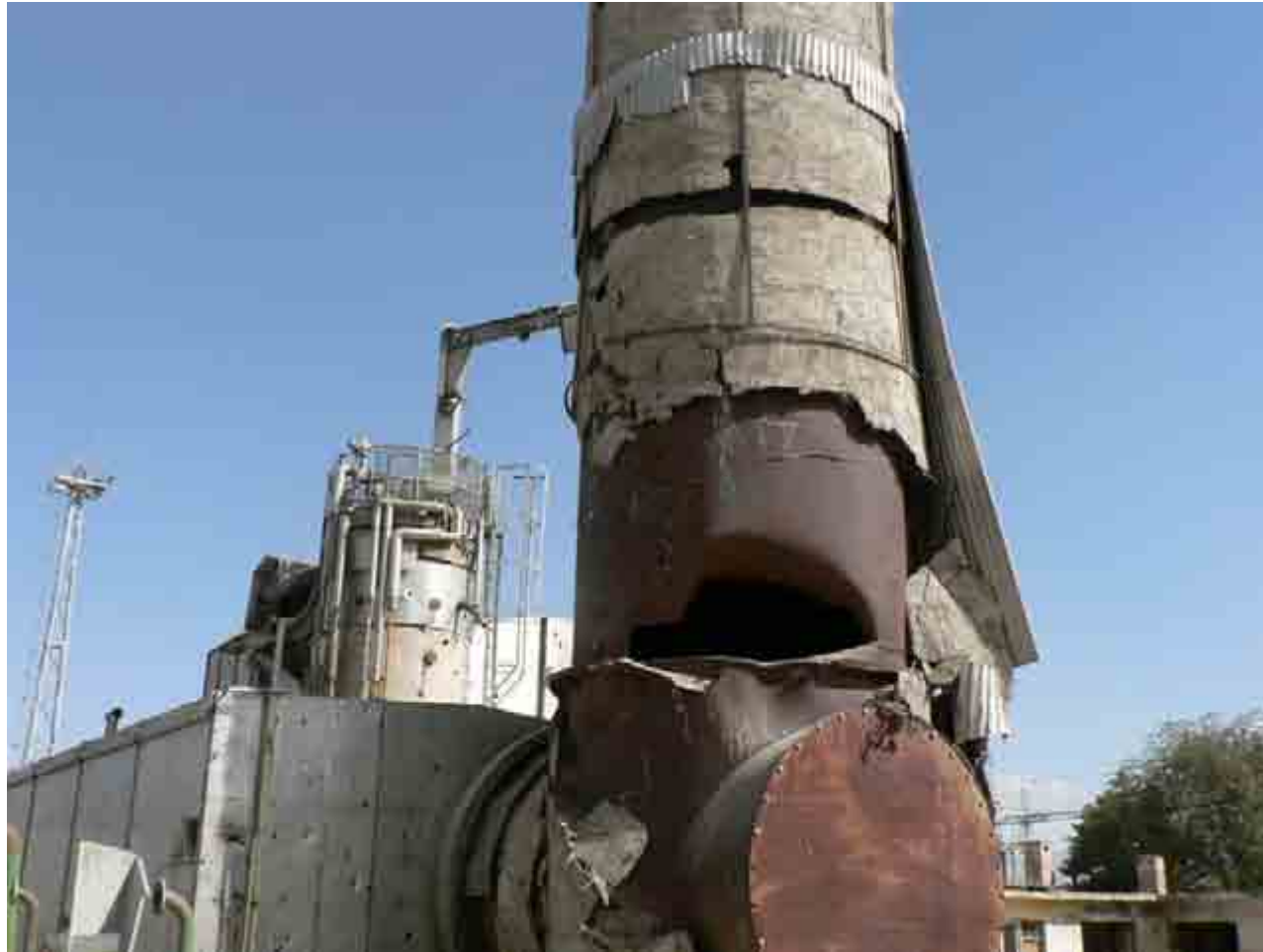
Figure 3: Kabul East Thermal Power Plant Damaged (Un-operational)
