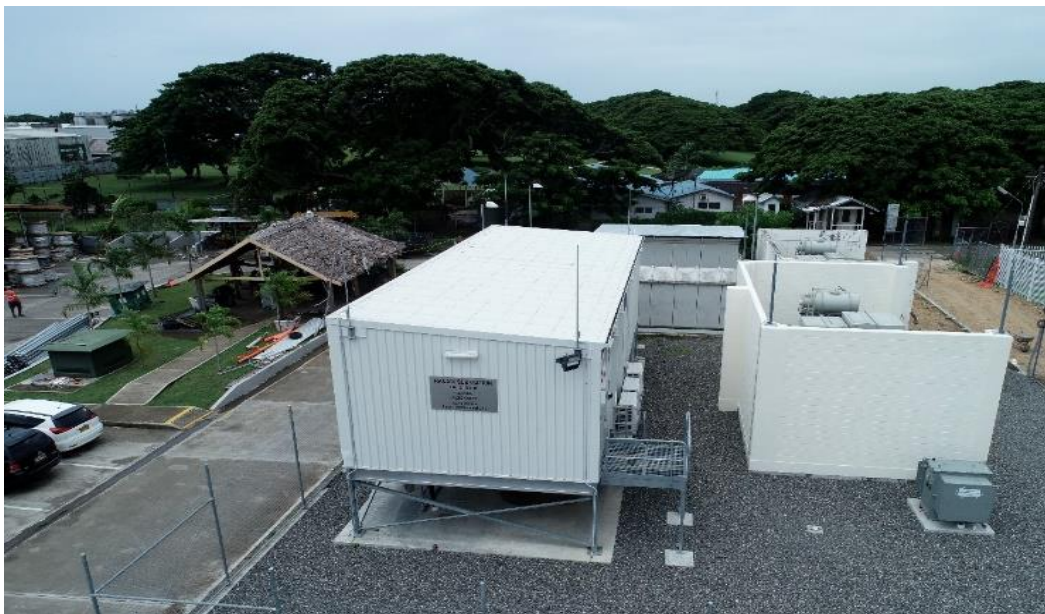
Ranadi Substation after upgrade
