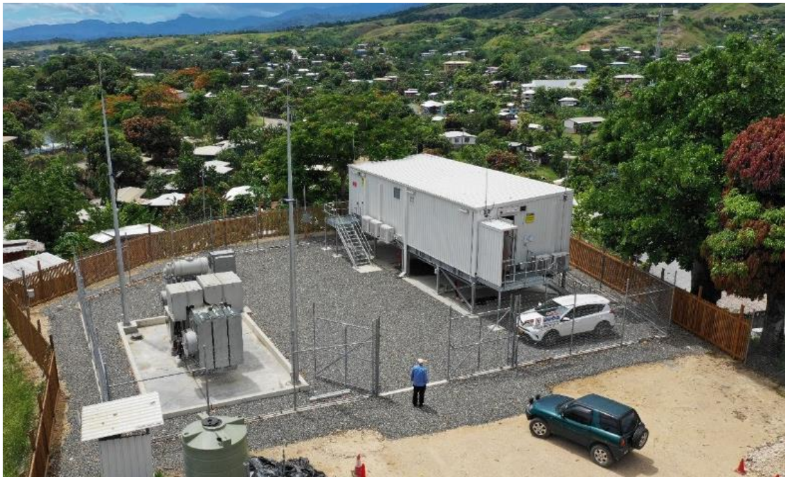
Kola'a Ridge Substation after upgrade
