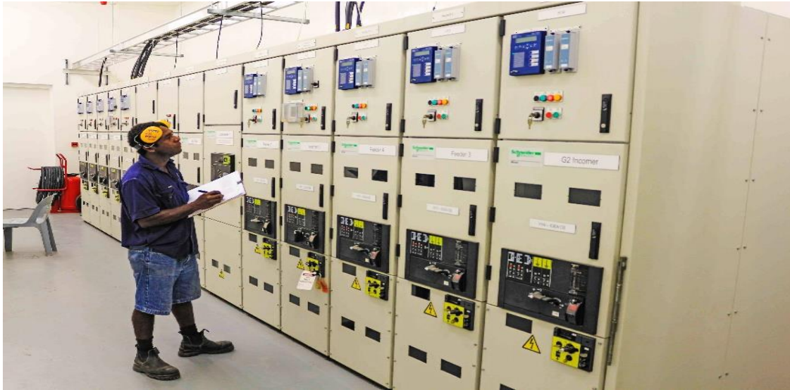
11 kV switchboard at Honiara Power Station
