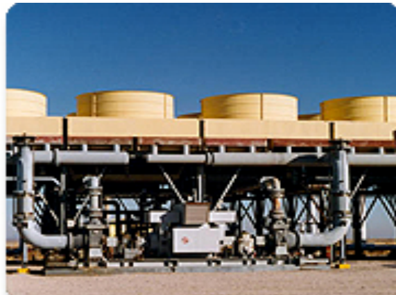
This geothermal power plant in Nevada has a capacity of 12 megawatts. Credit: Joel Renner, INEEL
